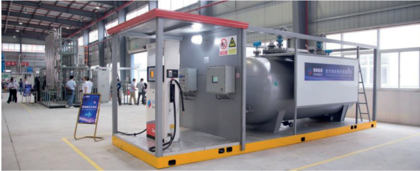
Figure 5. LOHC test station photograph (Muthukumar et al., 2023)
