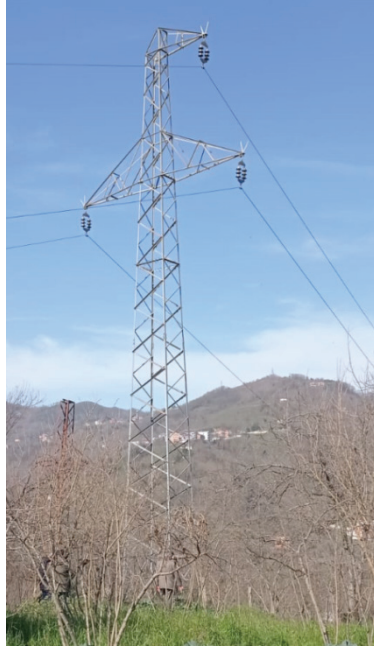
Figure 11. Galvanized bolted iron poles with 3/0 AWG (Pigeon) conductor used in MV
