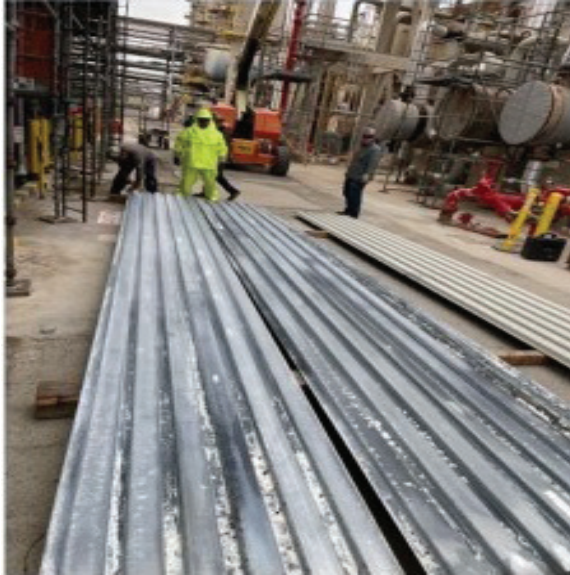
Figure 2. Example of White Rust on Galvanized Steel in industry (metaldecking.com, 2023).
