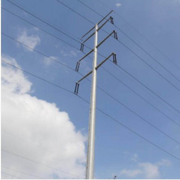
Figure 15. Tubular iron (galvanized) poles [1]
