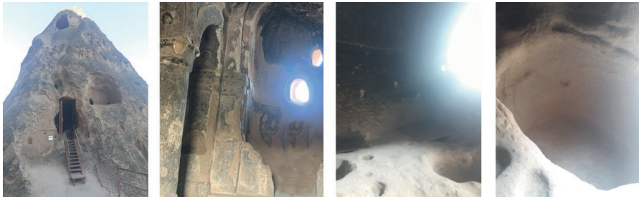
Figure 8. Anthropic deterioration of Aksaray Selime Cathedral
