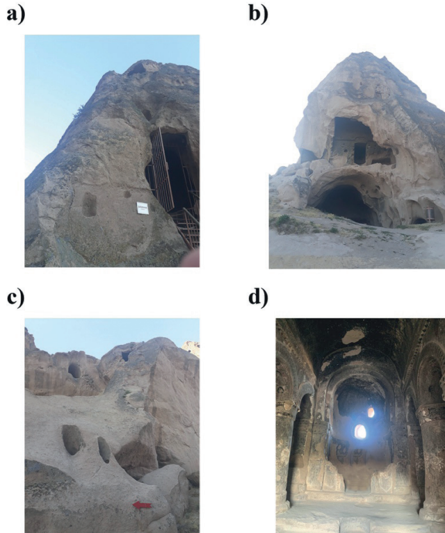
Figure 5. Physical deterioration of Aksaray Selime Cathedral
