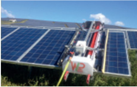
A) Wash Panel
